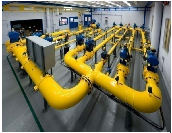
The closed high pressure test loop at FortisBC in Penticton BC, Canada
